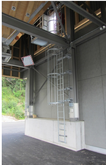
Double module silo with photovoltaic system
