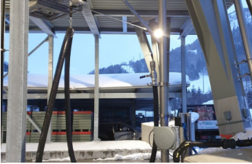
Mobile electric conveyor system for returning salt from the gritting silo in Airolo
