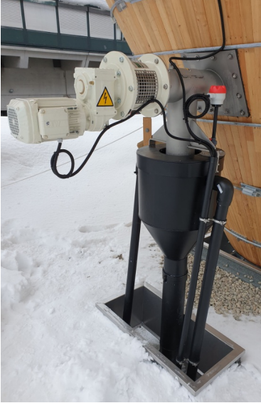
Brine generator with salt dissolving system and storage tank with mixing station
