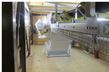
Loading facility of the grit silo plant
