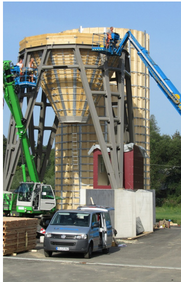
Loading by belt weigher at the silo hopper at the gritting silo facility
