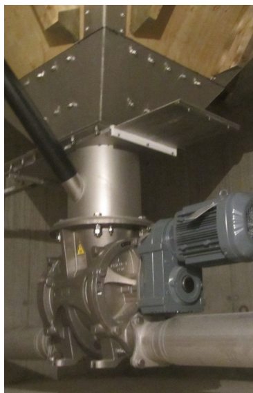
Technology of the silo plant in Bern Wankdorf
