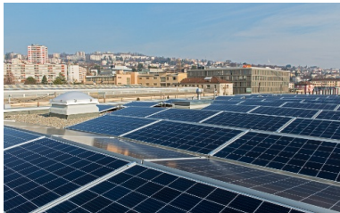
The photovoltaic system on the roof of the temporary office building supplies it with energy.
